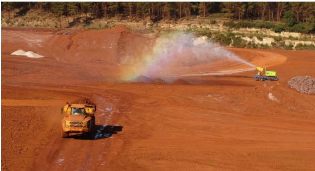
Figure 2. Watered track for the traffic of dumpers on the left of the image, and mist cannon in the background.
